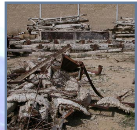
Opornaya gas compressor station shop demolition staff health hazard from asbestos containing waste
