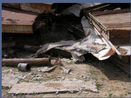
Worker exposure to asbestos during a gas compressor station shop demolition
