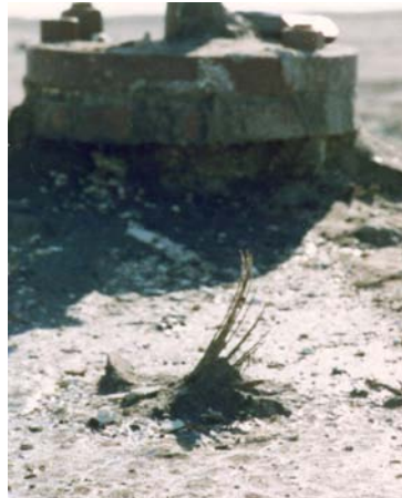
Bird trapped in seeping oil at a incorrectly shut wellhead
